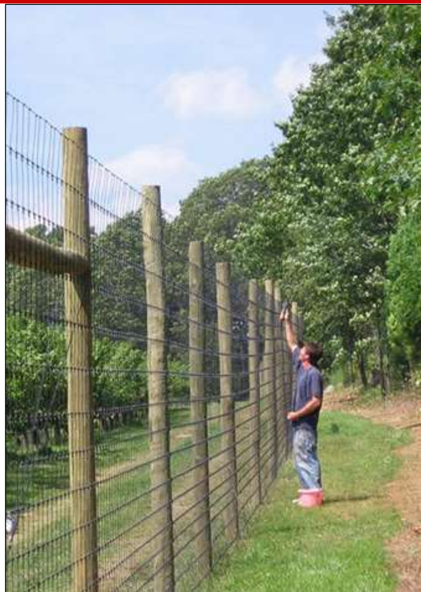
Wire Mesh Fencing
